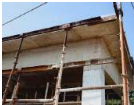
Finished surface of the single storey structure cast with the geopolymer concrete
