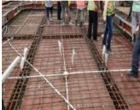
Arrangement of reinforcement and embedded strain gauges in slabs and beams of single storey RGC structure
