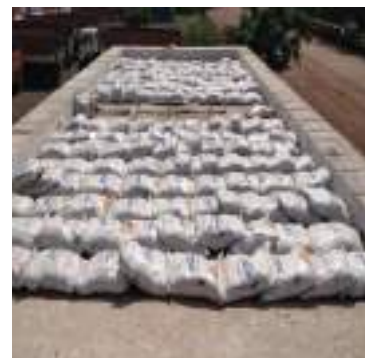
Arrangement of load on the slab using sand filled bags for load testing
