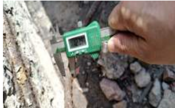
Measurement of existing rebar diameter of an RCC member at a Building site
